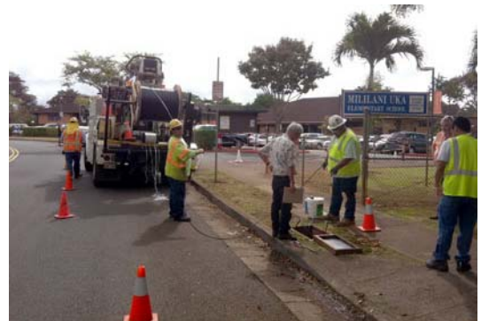
Members of a construction crew lay fiber to connect Mililani Uka Elementary School in Mililani Town, HI
