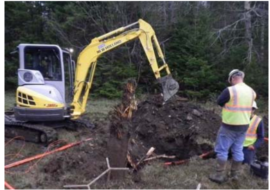
ION crew members clear a path to lay new fiber for its 1,300-mile project in upstate New York.
