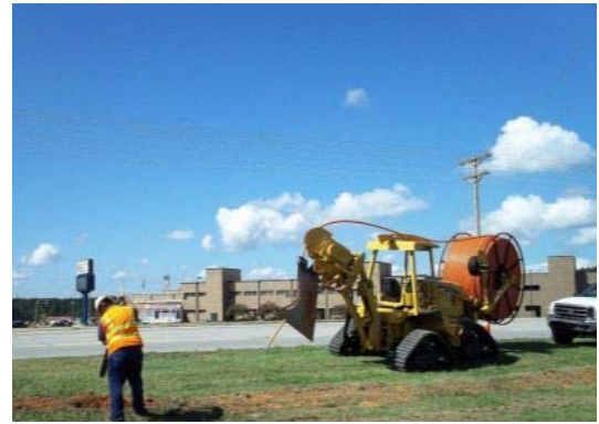
A construction worker in Walhalla, S.C., deploys fiber to connect a local school to the new Oconee County high-speed fiber network.
