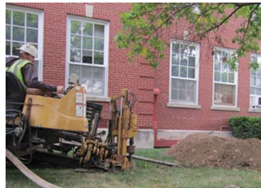
A member of an MUFN construction team drills a hole to install fiber.
